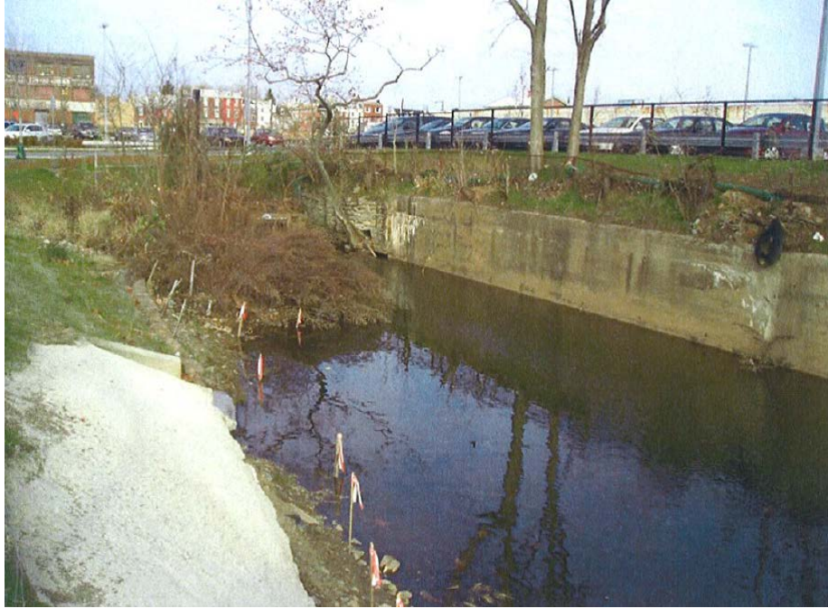
Looking northwest at the head of the Shackamaxon Street Drainage Channel and the existing brick sewer outfall
