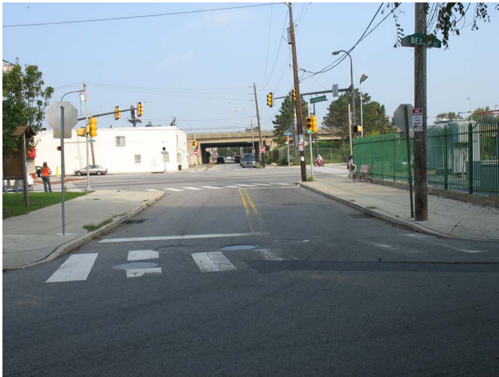
Figure 1: Deteriorated pavement markings at Columbia Avenue and Beach Street
