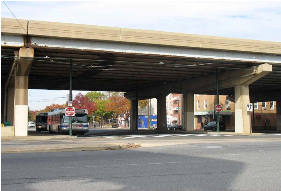
Figure 4: Missing guiderrail around I-95 pier at Cumberland Street and Richmond Street intersection
