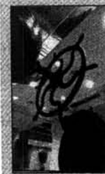
An exterior water valve (left) and huge condenser are now ornamental features in the building.
