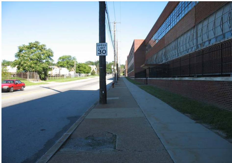
Figure 1: Poor condition of sidewalk on Fox Street near site access
